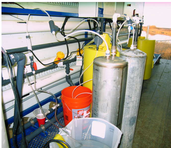
Figure 2. Photograph of the Calcite Filter Pilot System
